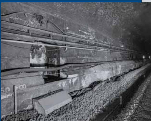
Ashlar granite walls and the overhead brick arch of the tunnel extension built between 1903 and 1906, and the electrification cables installed in the 1930s characterized the tunnel interior in the late 20 th century. One of the round-arch worker safety niches is shown in the north wall which provided workers a safe location to wait while trains passed. (2014)
