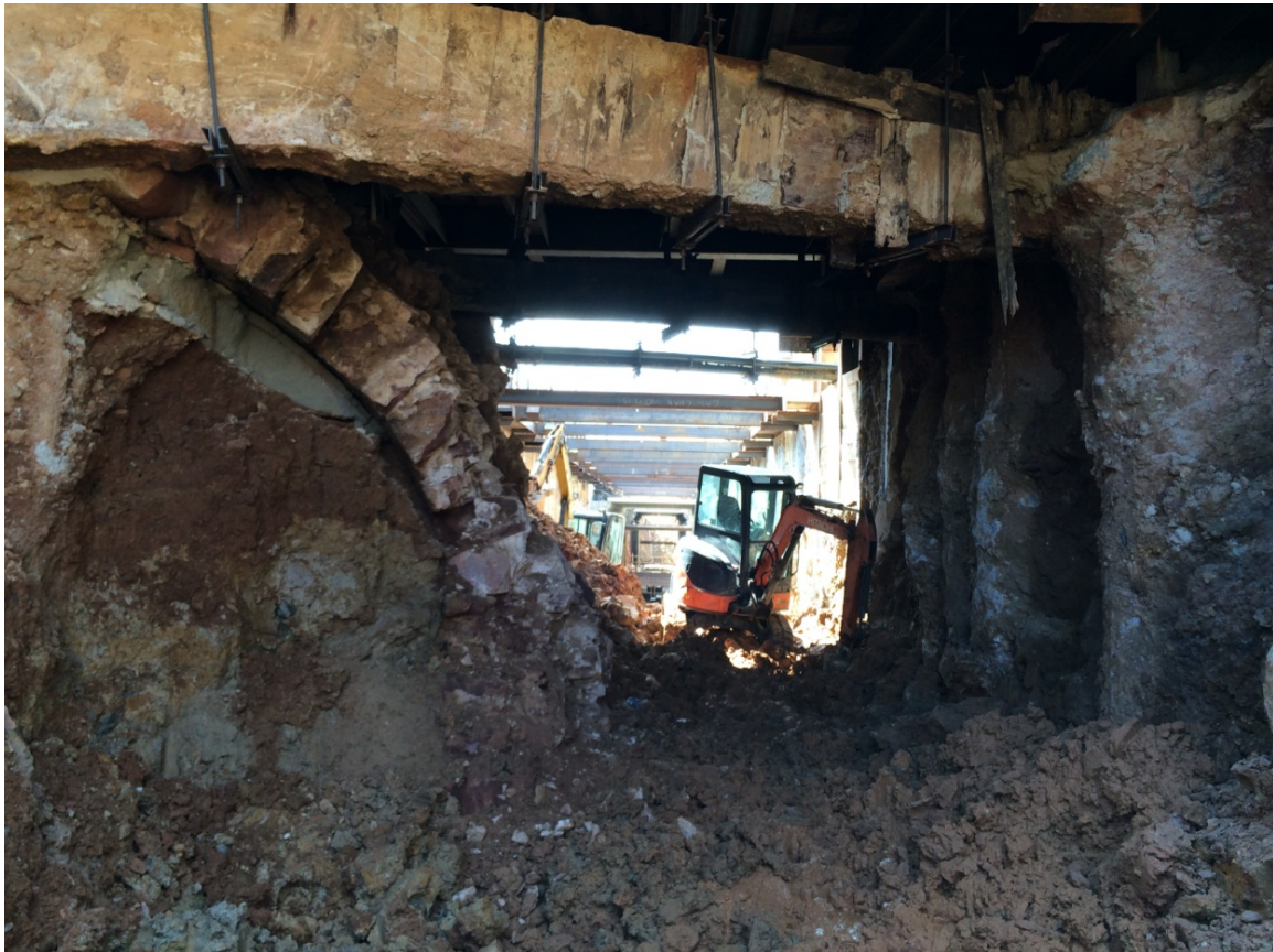
The abandoned segment of the 1872 Navy Yard Tunnel at left, under 7 th Street SE, looking west/northwest.
