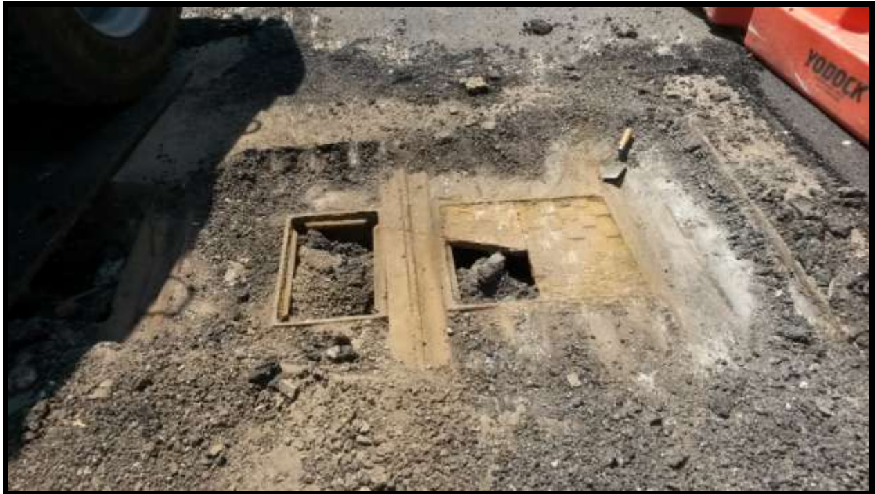
Streetcar slot and wheel rail and access panel frame (VAT-2015-HB-001) on 8th Street SE, looking south
