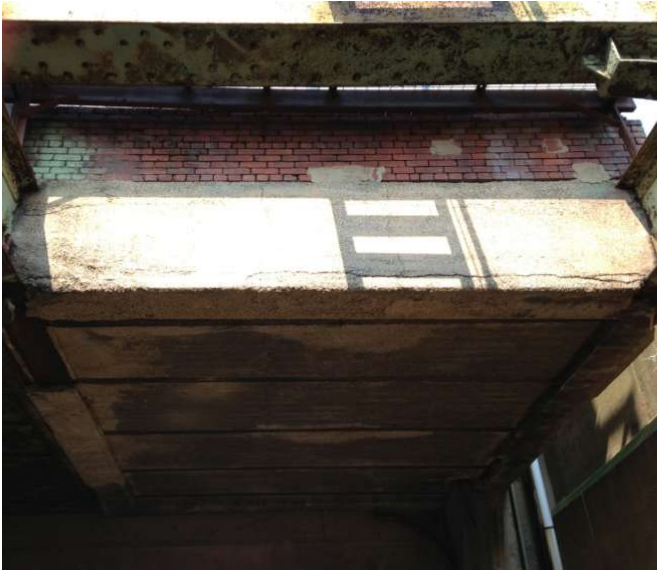
Figure 2. Steel girder and concrete platform under Control Point Virginia Tower and its exterior basement wall.
