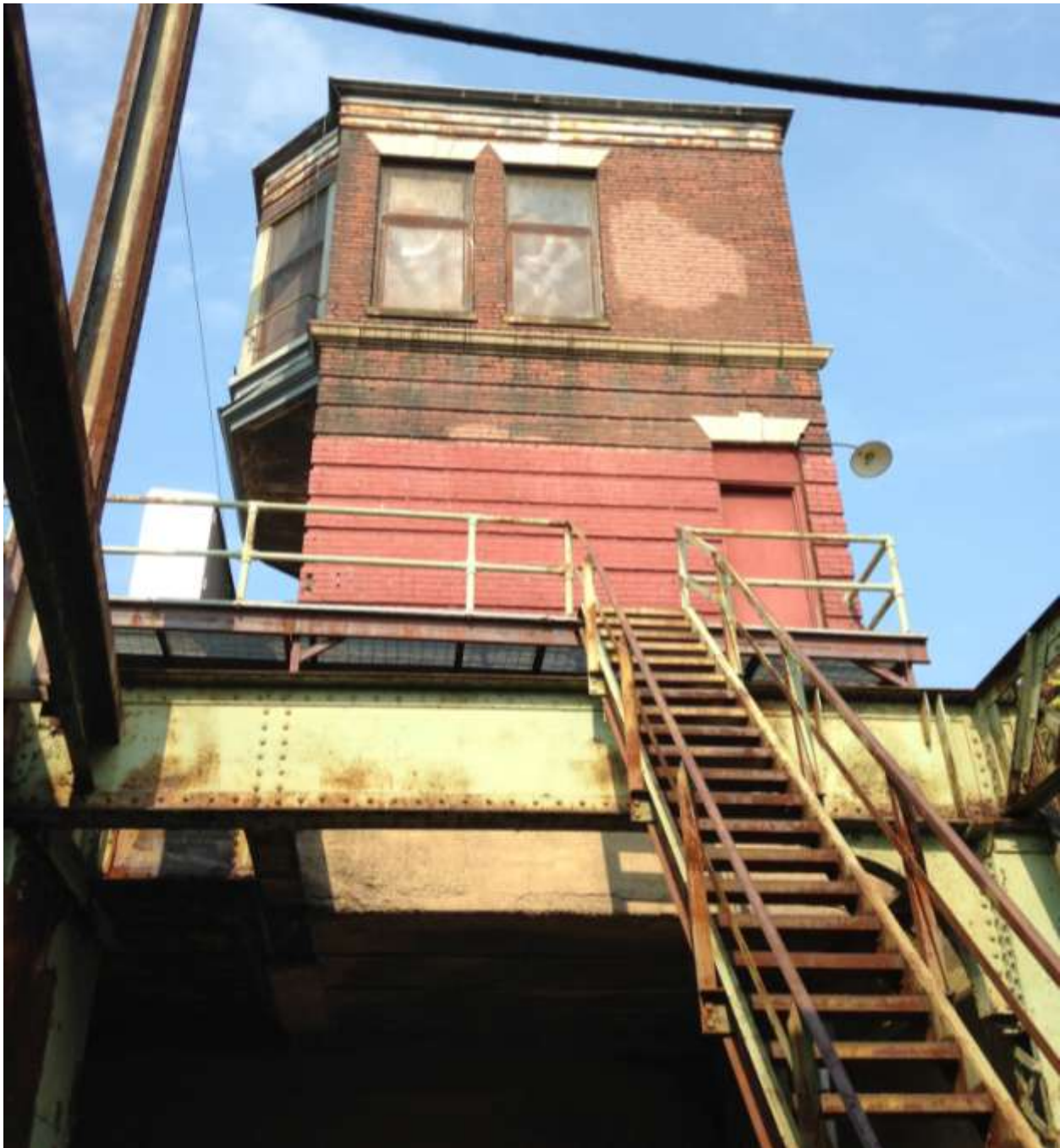
Figure 3. Steel staircase attached to steel platform on the East Elevation, Control Point Virginia Tower.
