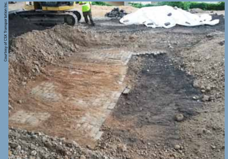
Intact segment of cut granite block pavers from Virginia Avenue SE found under the 11th Street SE Bridges. The road is about 20 feet wide. Removed paving stones are piled in the background and were donated for reuse by the District Department of Transportation.
