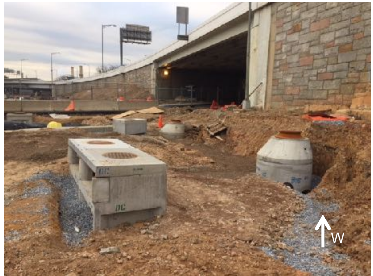
Street Drainage Infrastructure
